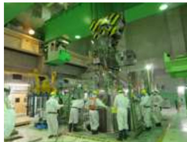
Fuel removal work at Fukushima Daiichi NPS Unit 4 (Cask transfer at common pool) @TEPCO
