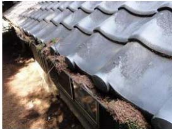
Rain water gutter (before)
