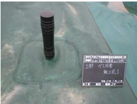
Methane gas venting pipes generated during storage of combustible materials
