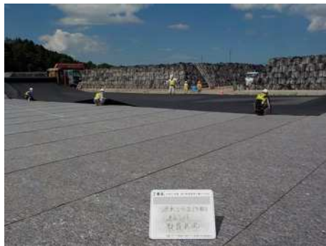
impermeable liner sheet installed at the bottom of the temporary storage site.
